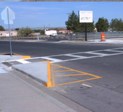
a. School zone sign b. Bicycle parking at Mesilla Elementary c. Crossing improvements at Valley View
